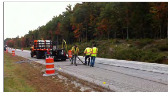
DISPENSED AT OVER 350 DEGREES THE RUBBERIZED ASPHALT SEALANT IS INJECTED DIRECTLY INTO THE PAVEMENT CRACKS
