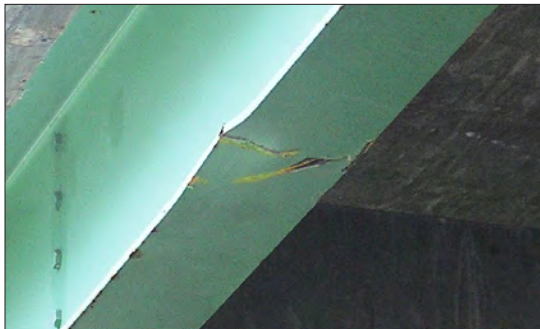
GODDARD ROAD SB OVERPASS, MILE 79.6, 2013 BRIDGE HIT WAS REPAIRED BY CONTRACT IN 2014
