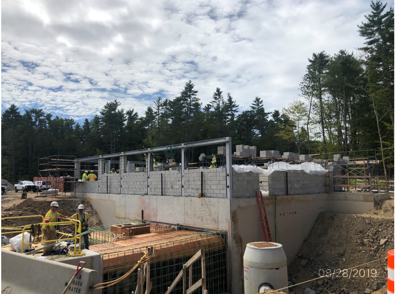
The cast in place connector from the tunnel to the toll building.
