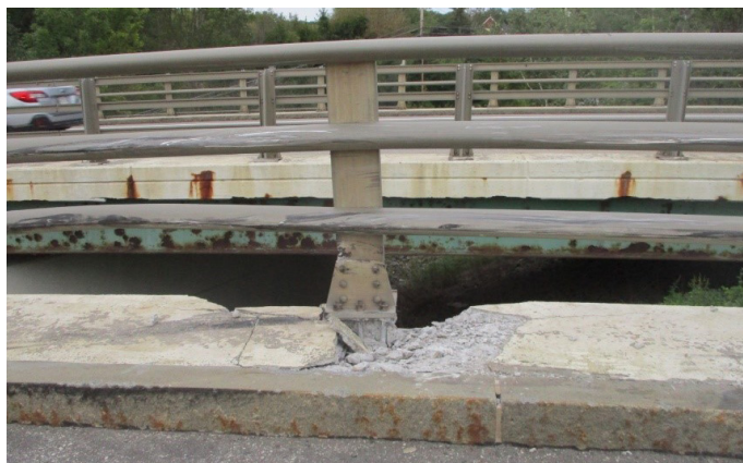
CENTRAL STREET OVERPASS BRIDGE RAIL DAMAGE
