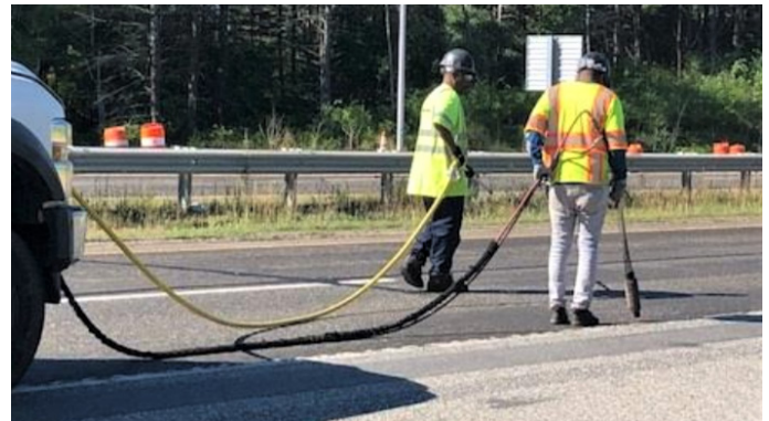
DISPENSED AT OVER 350 DEGREES THE RUBBERIZED ASPHALT SEALANT IS INJECTED DIRECTLY INTO PAVEMENT CRACKS DURING CRACK REPAIRS
