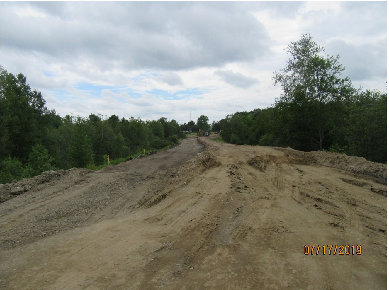
Removing gravel from the old ramp to the new access road elevation
