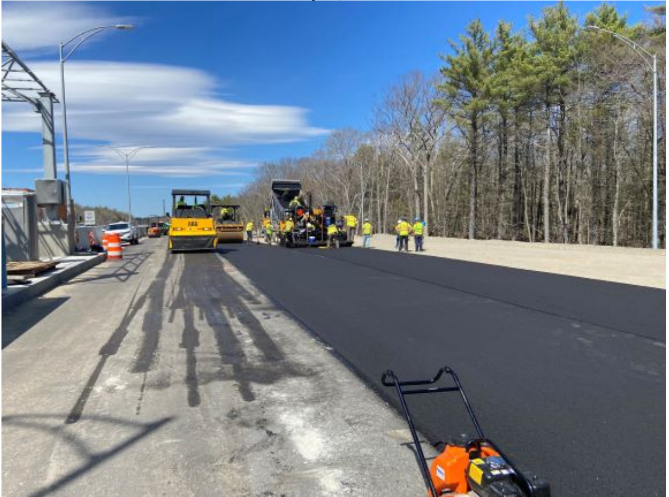
Pike's paving crew paving the north bound cash lanes, north of the new plaza, looking north.
